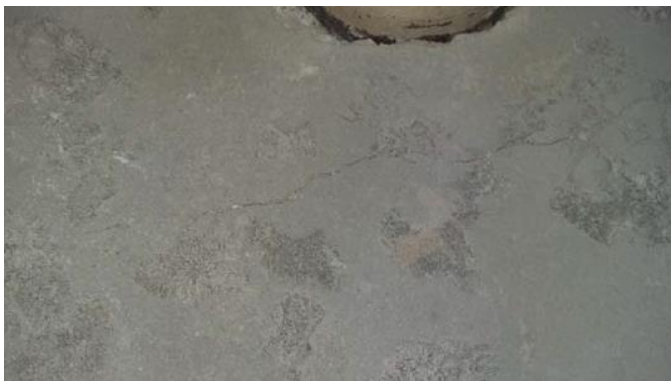
Figure 2: Cracks in the building
